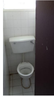
Image 44 - Toilet linked to sewer (Region 3)
